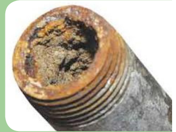
Corrosion buildup in galvanized plumbing can severely inhibit water flow.
