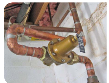
PRVs are commonly installed either near your water meter or water tank (pictured above)
